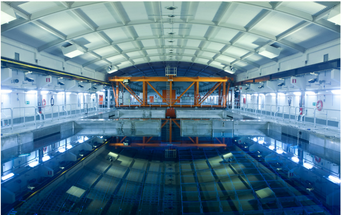
Figure A4 Storage pool in Clab. The top edge of the spent fuel is eight metres below the water surface.
