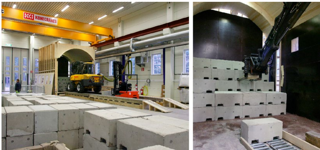
Figure A5 The Multi-purpose Test Facilities at Äspö. The photo shows the testing of a self-positioning robot for backfilling a deposition tunnel with bentonite blocks.
